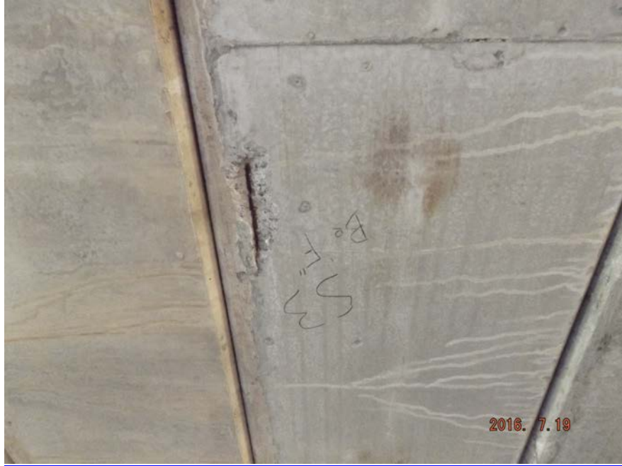
SPAN 3 - BEAM F - REBAR SPALL
