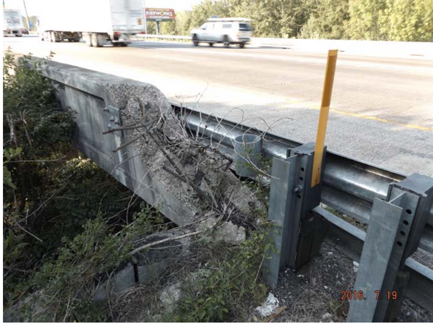
APPROACH 2 - RIGHT - RAIL DAMAGE
