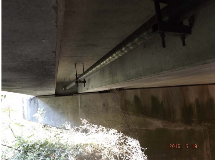
ATTACHED TDOT FIBER
