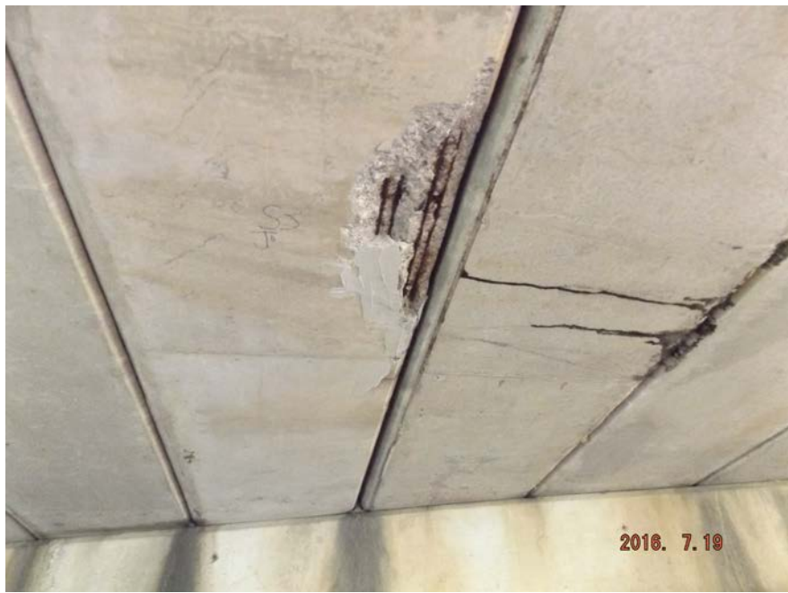
SPAN 3 - BEAM J - REBAR SPALL
