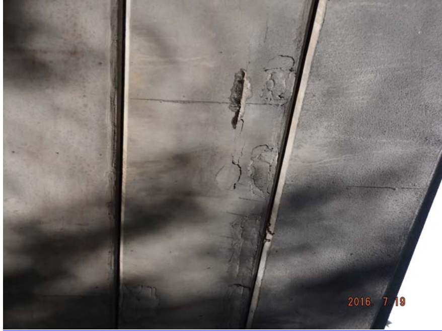
SPAN 2 - BEAM B - REBAR SPALL
