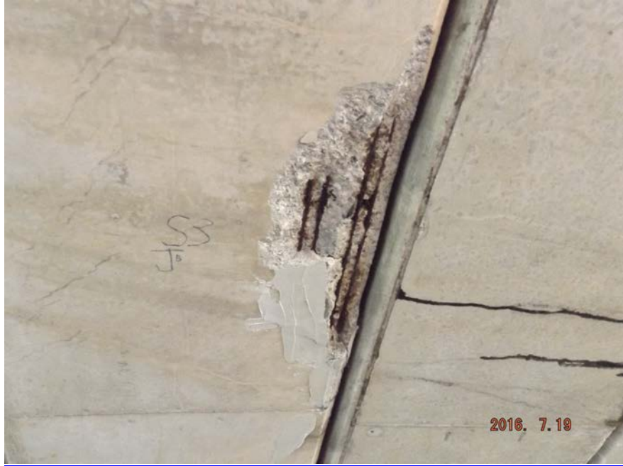
SPAN 3 - BEAM J - REBAR SPALL
