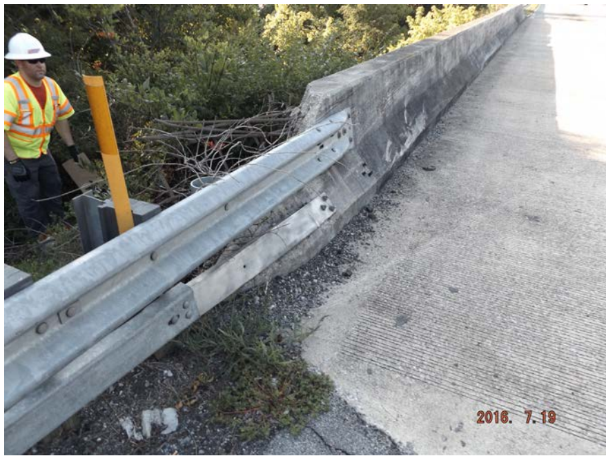
APPROACH 2 - RIGHT - RAIL DAMAGE
