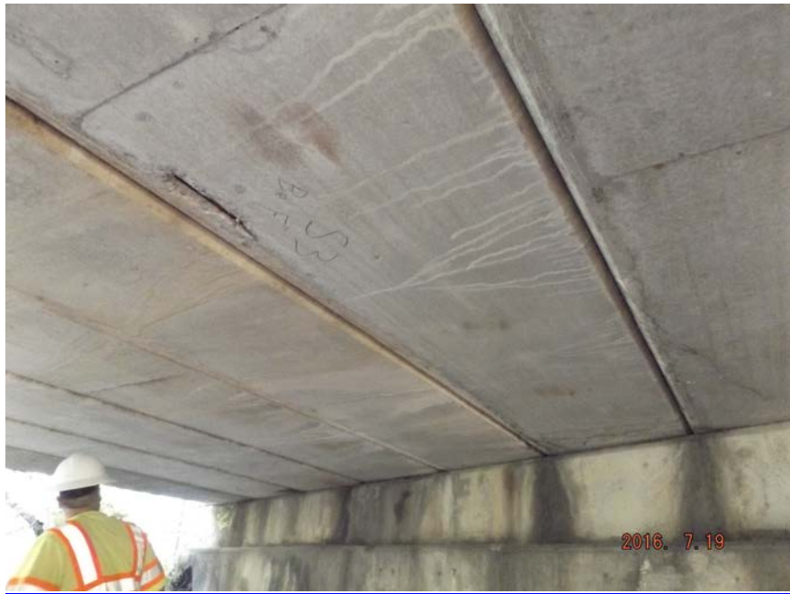
SPAN 3 - BEAM F - REBAR SPALL
